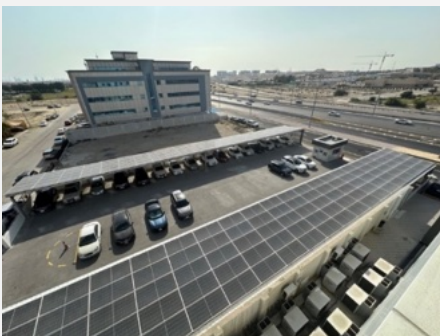
Solar carport powering KSA HQ lights
