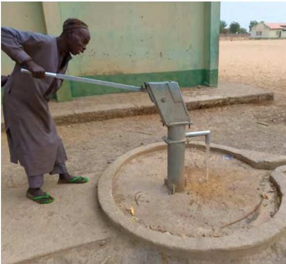
Establishing a Borehole in Tsintsiya Village, Nigeria, to Provide Access to Clean Water
